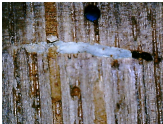
Figure 3. Timber pest passages within the wood
